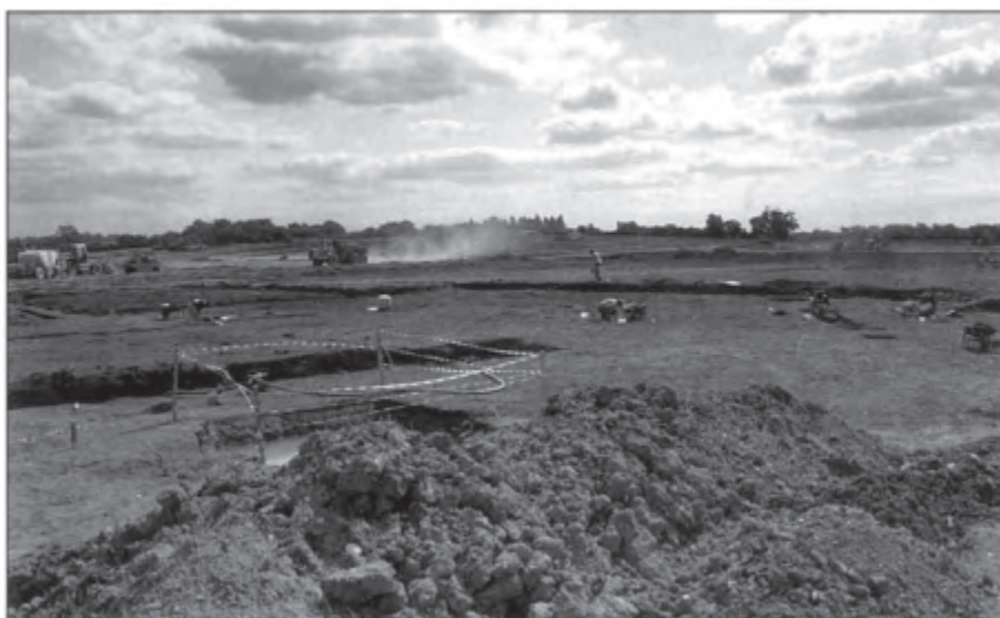
The south-eastern part of the site, looking east, with construction activity in the background.
