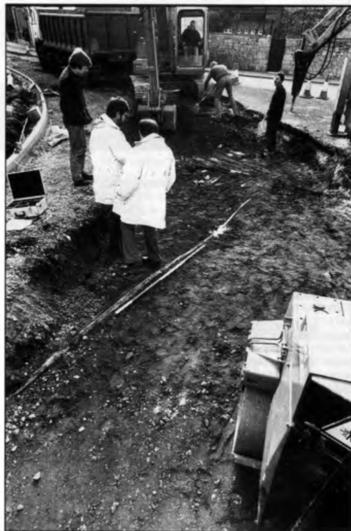
▲ The 3in. diameter lead waterpipe, exposed during roadworks close to the Military Road - Broad Street intersection
