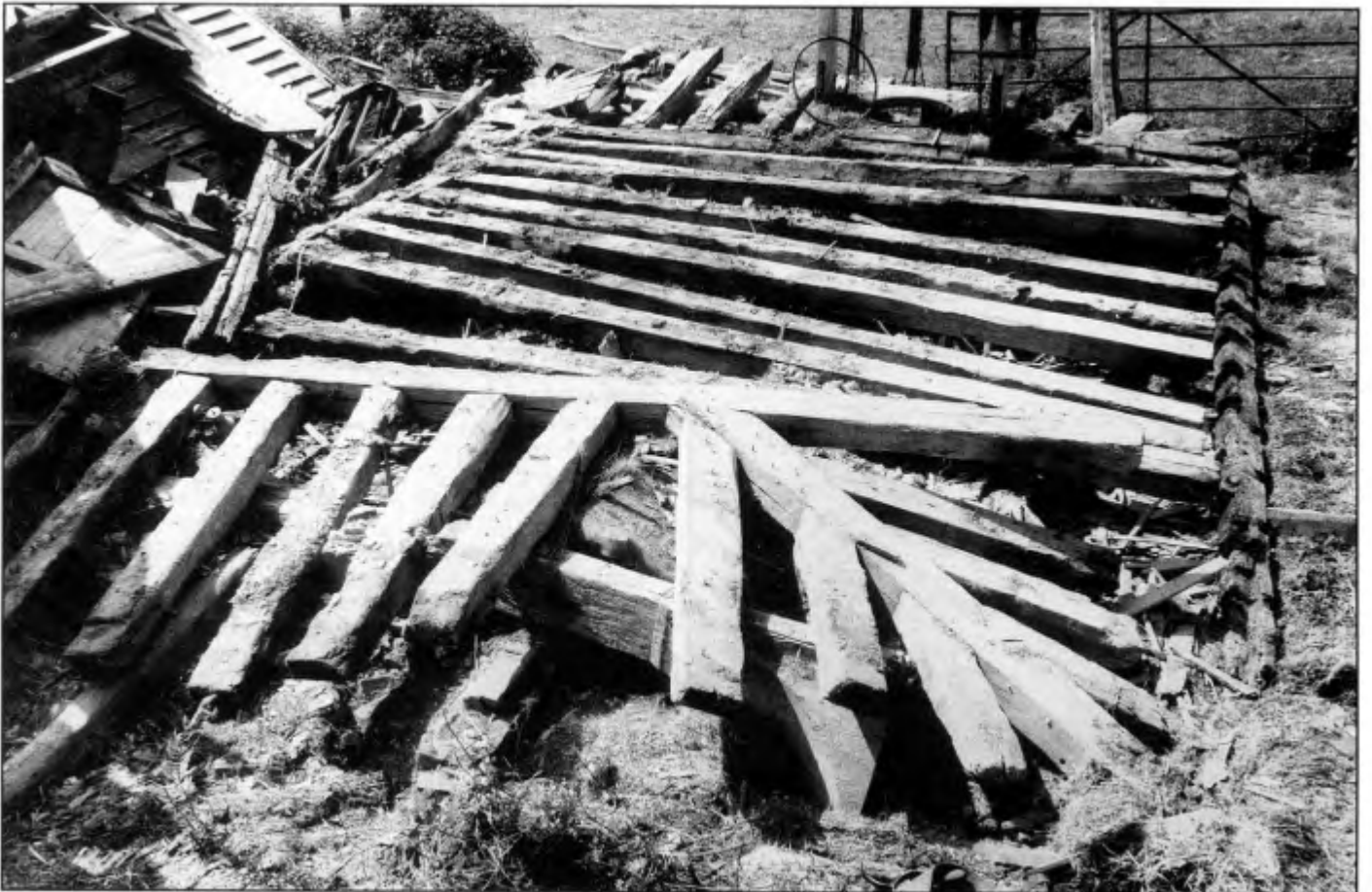
▲ Romden Hall House: solar first floor joists and dragon beam looking south-west
