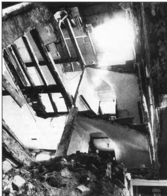
▲ Void left by collapsed stack
