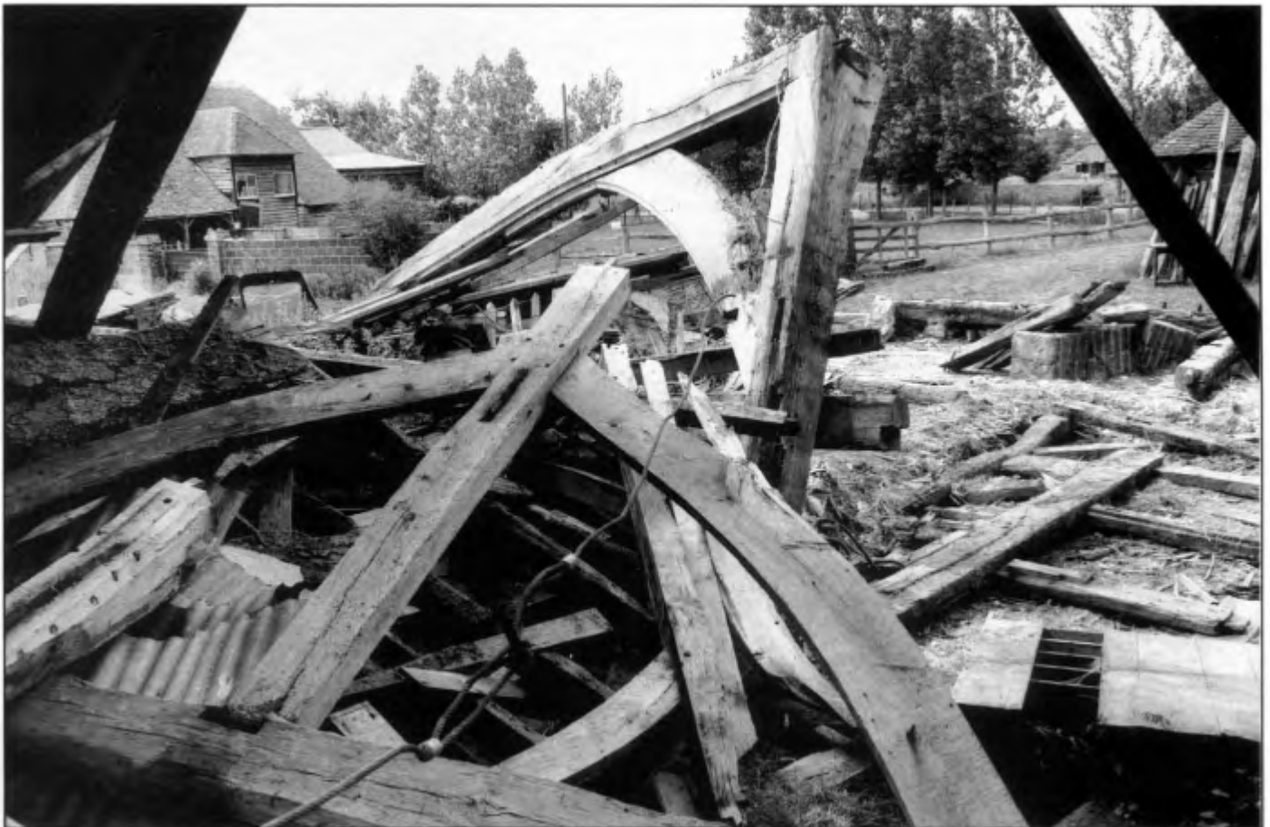
▲ Romden Hall House: collapsed remains of open hall looking west.
